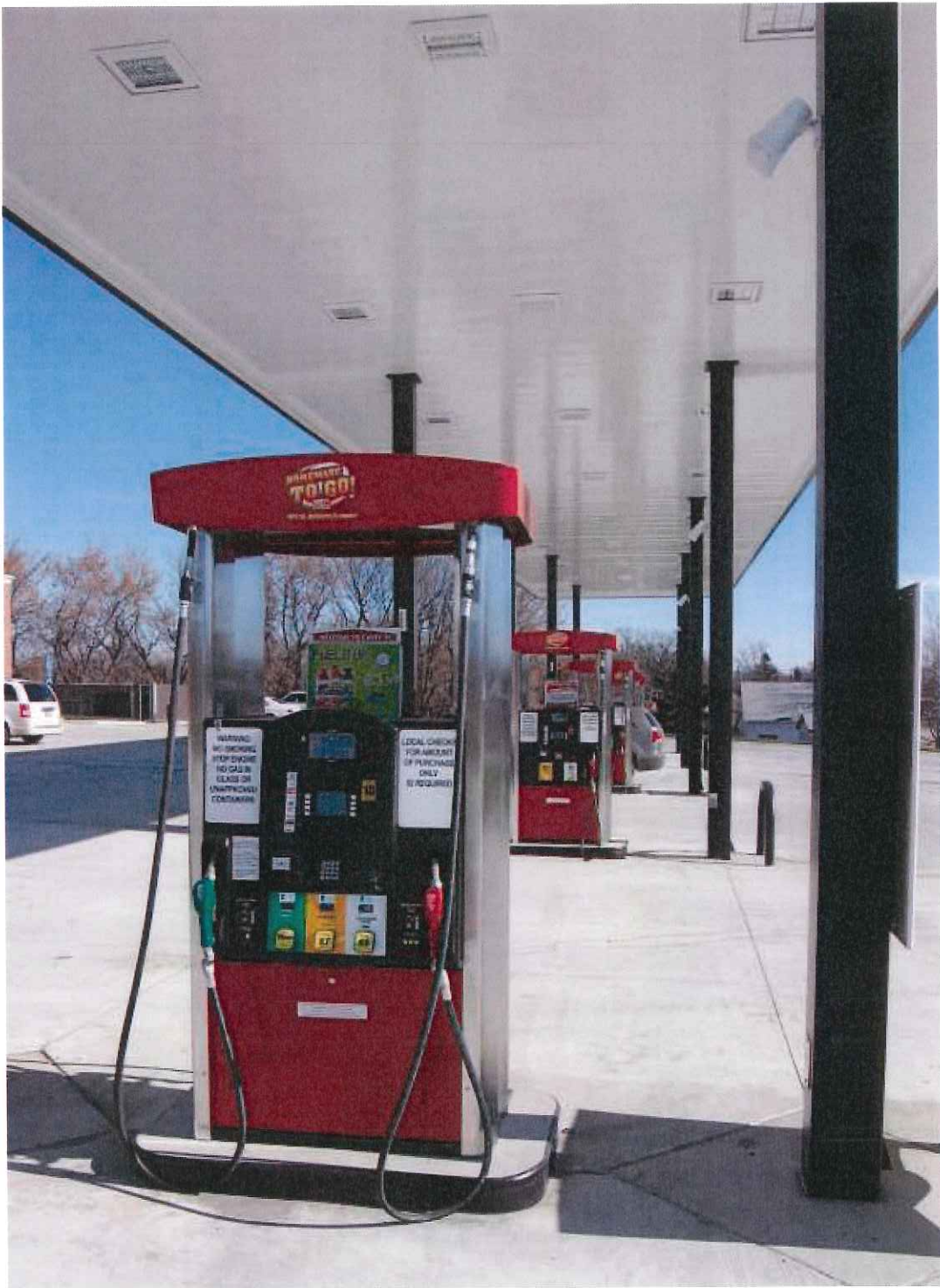
Typical Pump Signage
