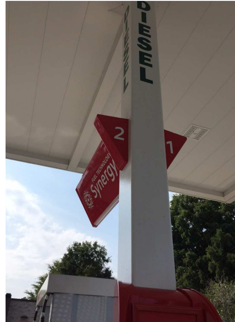
RE-BRAND: PUMP ID PANELS
