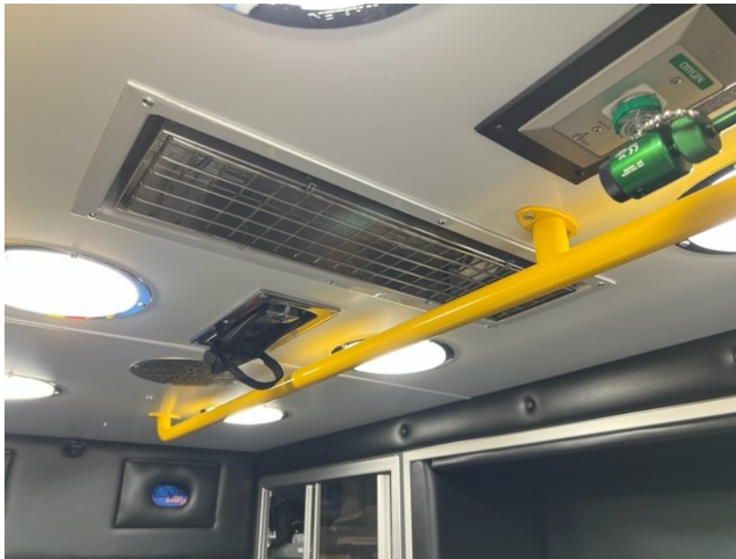
Ultraviolet light in ceiling of ambulance (behind wire cage).
