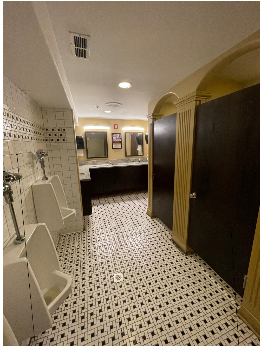
Remove wall tile. Patch & repair walls. Prepare for new wall tile in brick bond pattern
