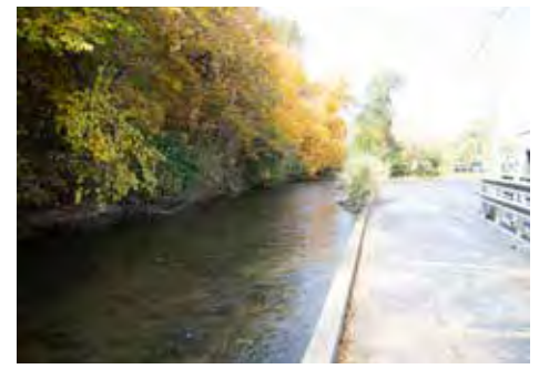
Eroded banks along Crystal Creek Reach 9 (CCR9)
